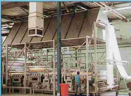
Vapour extraction installation
