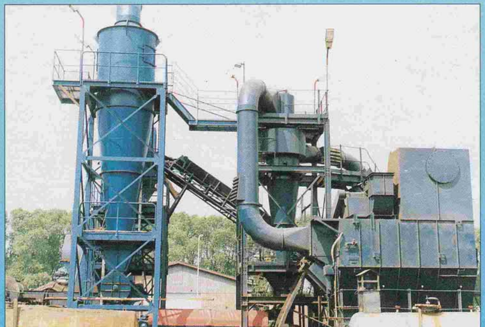
Cyclone erected in a shredder installation, removal by rotating air lock with a diameter of 1000mm. Fan B 33, capacity 46,000 m 3 /h. Total height of installation: 14 metres.
